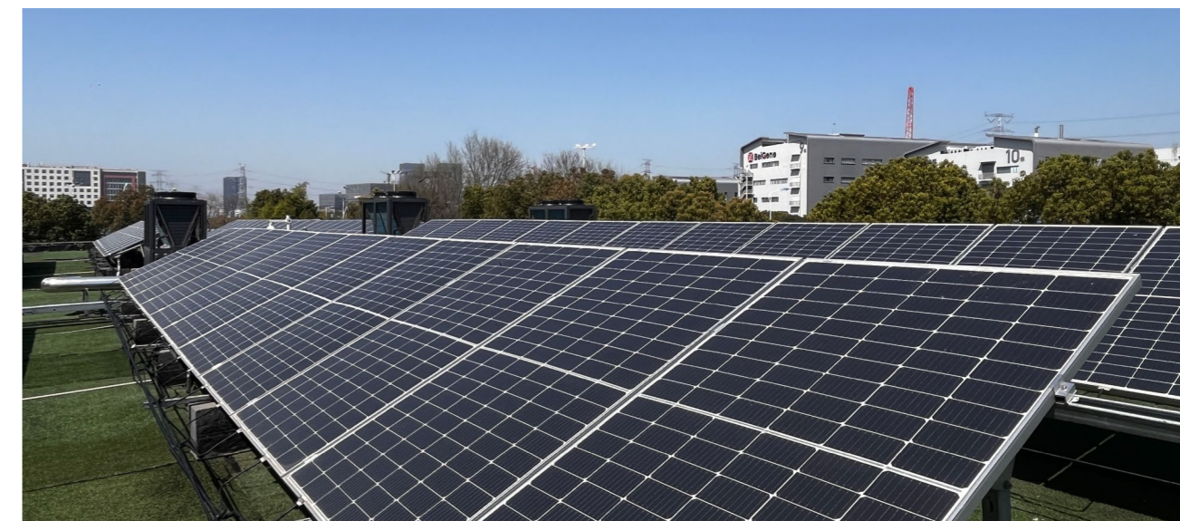
GCL Academy (restaurant) adopts photovoltaic thermal heat pump system (PVT)
